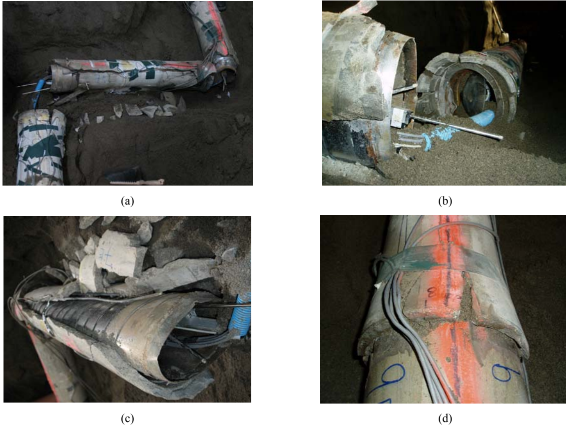
Fig. 7. (a) Excavated pipeline after PGD. Central pipe segment #7 was completely removed from segments #6 and 8. (b) The joint between segments #7 and 8 with LVDT needle evident. (c) Oval distortion of segment #7 due to extreme shear forces during PGD. (d) Telescopic failure at the connection between segment #8 and #9.
