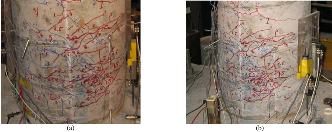
Figure 4 – (a) Crack pattern at 4% drift at the base (b) Crack pattern at 10% drift at the base
