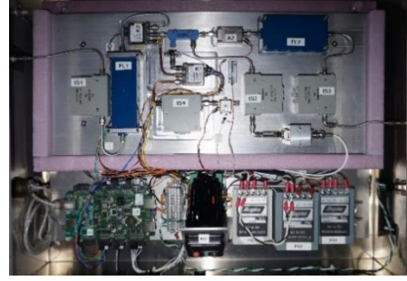
Fig. 5. LNA and calibration subsystem implemented on the PID controlled thermal plate
