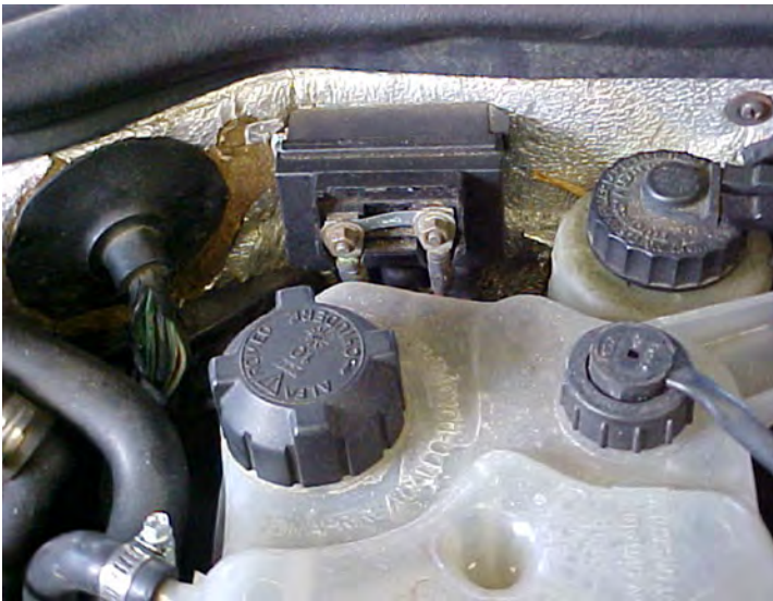
40-amp fuse at the firewall
