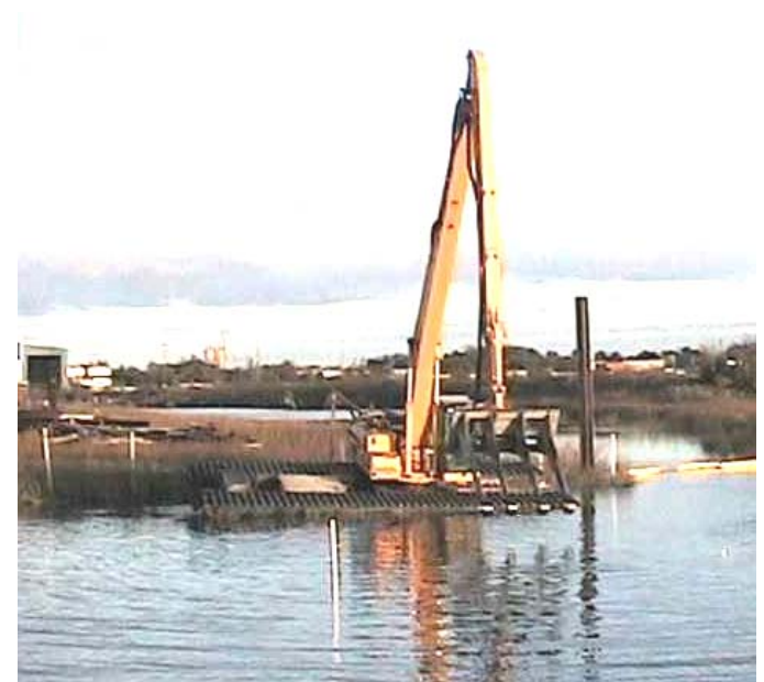
Injection System (Williams Environmental)
