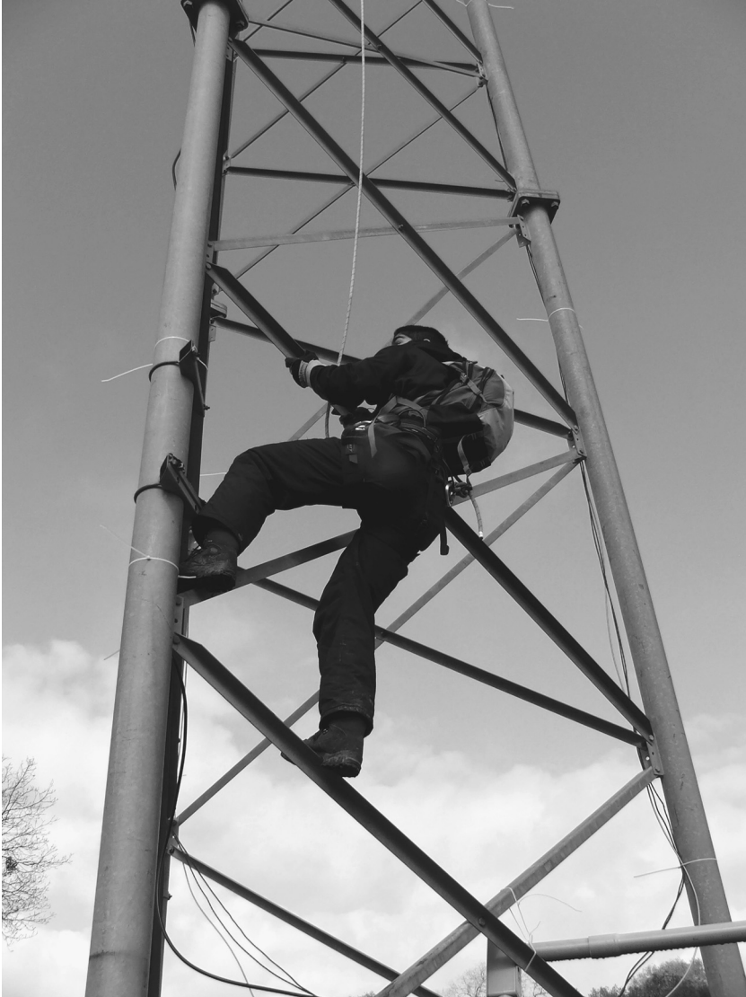
Figure 8.2 Joseph climbs a backbone tower on the Santa Ysabel Indian Reservation to the height of a seven-story building. Matt comments, “We didn’t get all the safety equipment that comes with these towers . . . like the ladders.” (2006)
